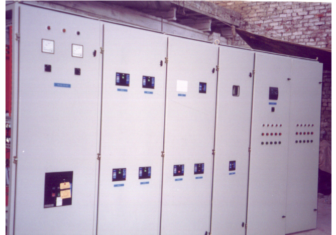
(Main L.T Control Panel))
