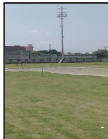
Construction of Hockey Ground and Installation of Flood Light Poles in District Sargodha
